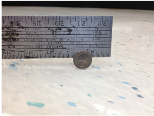
Subfloor out 1/2" in 12". Owner complaining about burnish marks
